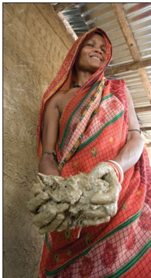
CRS project participant Sukanti Dalai uses an improved mixture of mud and straw to complete the walls of her home using techniques to make it more flood resistant in the village of Raipur in Orissa state. Dalai and her husband have lost their home to flooding more than a dozen times in their lifetime. • Photo by David Snyder for CRS
